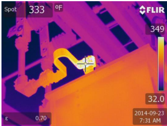
Figure 5. Voltage regulator near failure at a mine substation [13]
